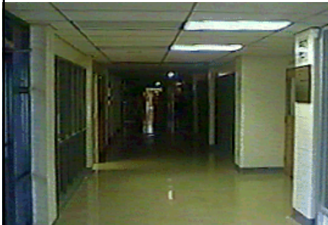
Above: The corridor in front of the main office lies in darkness at midday Tuesday. This portion of the first-floor hallway was one of several scattered areas in the building which lost power for about 78 minutes.
