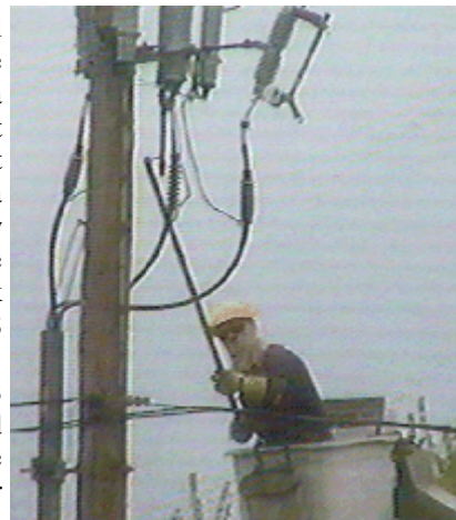
Above: A Connecticut Light & Power worker repositions an electrical connector at 12:21 PM Tuesday, restoring power to all of NHS.
